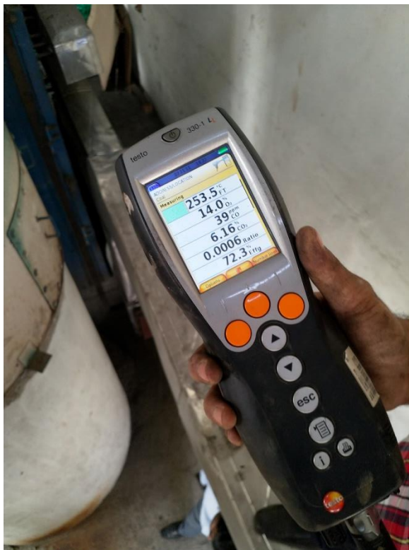
Figure 2: Flue gas analysis results at a unit
